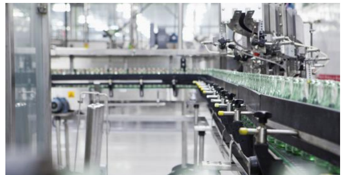
Figure 12: A company can establish fully-automated operations by implementing devices throughout the factory that acquire, communicate, and react logically to massive amounts of data.
